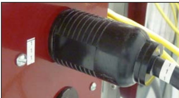
Element jumper cord properly installed:
